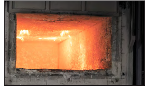
This stack heating device uses heat exhaust to preheat aluminum before it is melted, thereby conserving natural gas.
