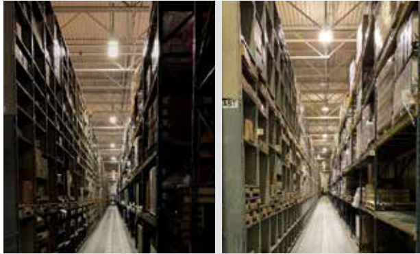
The image at left shows an aisle in the Mercury distribution center before the March 2021 project to replace its fluorescent high-bay light fixtures, and the image at right shows the same aisle after the installation of high-efficiency LED light fixtures. The project increased light levels in the warehouse by 36% while saving on energy costs. The project saves $12,000 each year, with $6,100 of the annual savings coming from reduced energy consumption and $5,400 from reduced maintenance and re-lamping costs.
